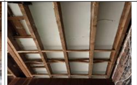
Potential asbestos in floor between joists to be tested
